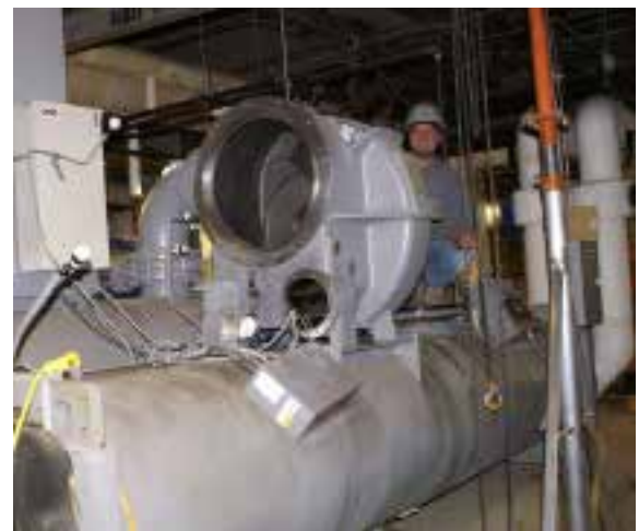
PMT Service Technicians perform field inspection and repair of a Carrier 19FA centrifugal chiller.
